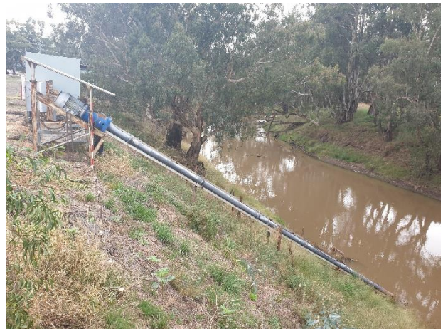
Figure 5-8: View east showing the banks of the Lachlan River and existing pump station facilities
