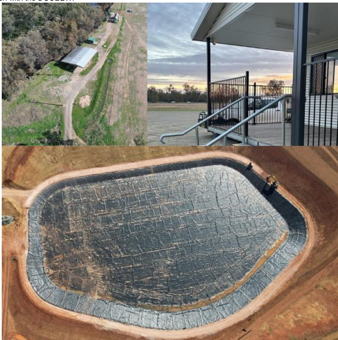
Top left: An aerial image of the LRP site at the location of the upcoming pipeline works; Top right: the completed LRP building; Bottom: A birdseye view of the raw water storage lagoon at the Parkes WTP.
