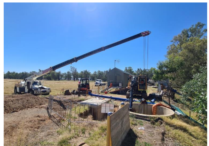
Augmentation of the Lachlan River Pump Station.
