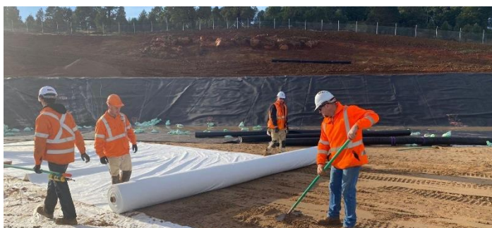
Installation of geofabric and liner on the RWSL floor at the Parkes WTP.
