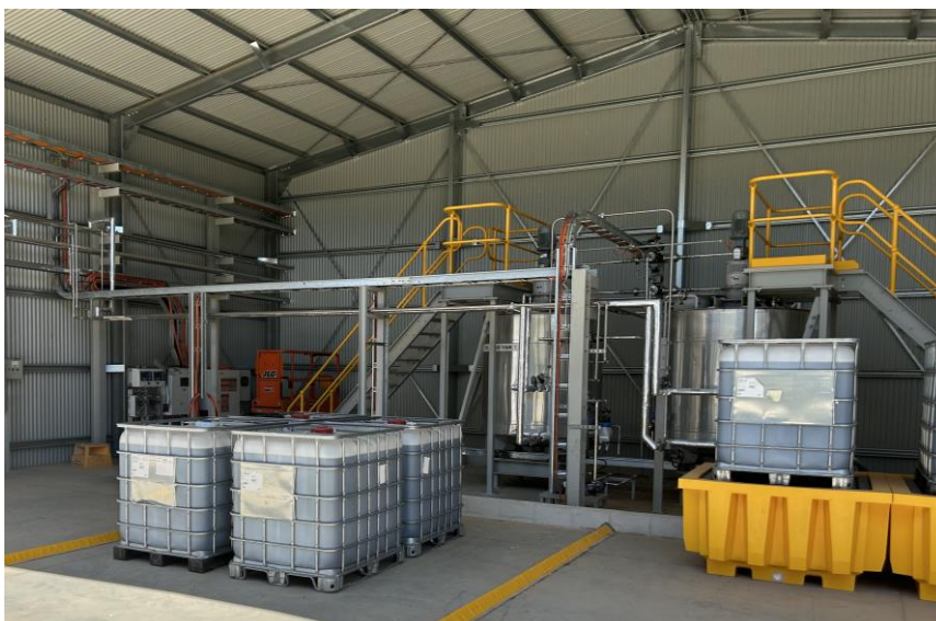
Figure 6: Fuel Blend Tanks
