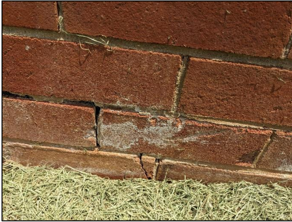
White staining at the base of the dwelling
