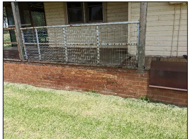
Base of dwelling presenting dampness "tide marks" and signs of mechanical breakdown due to salt crystals
