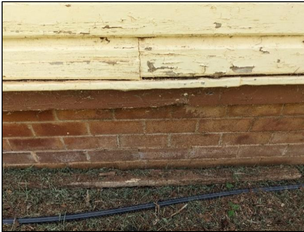
White staining due to salt crystals at the base of the dwelling
