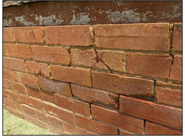
Brickwork presenting white staining and signs of mechanical breakdown due to salt crystals
