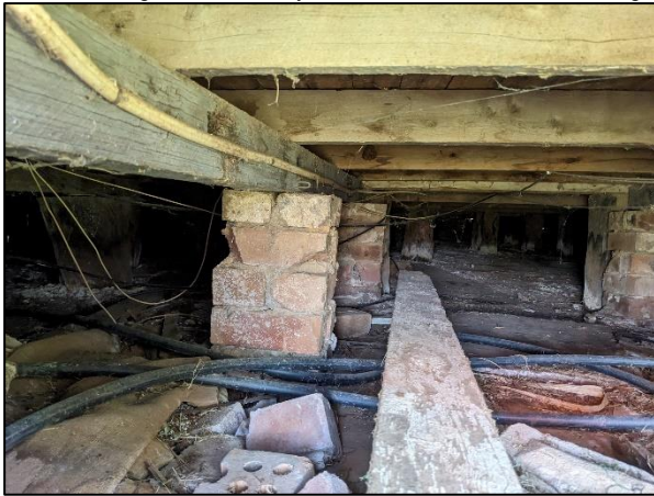
Footings presenting signs of mechanical breakdown
