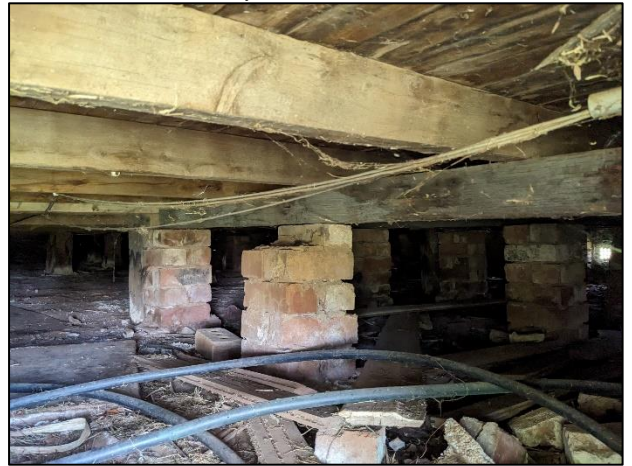
Footings presenting signs of mechanical breakdown
