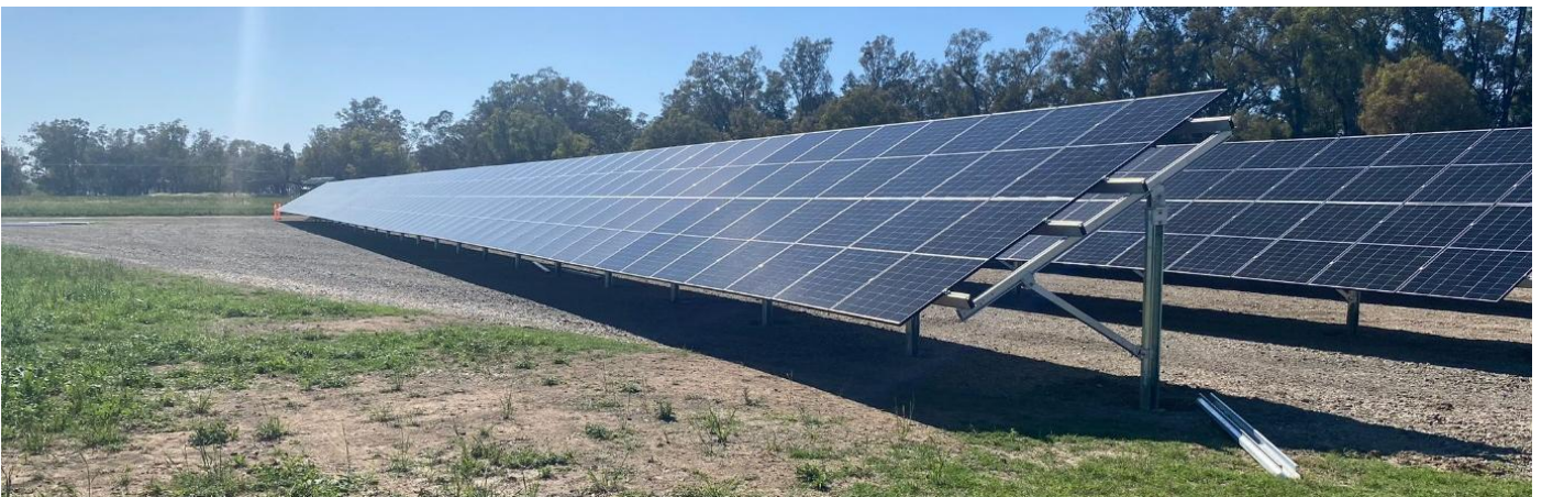
Figure 2: The new solar array at the Lachlan River Precinct will help power the Lachlan River pump station.
