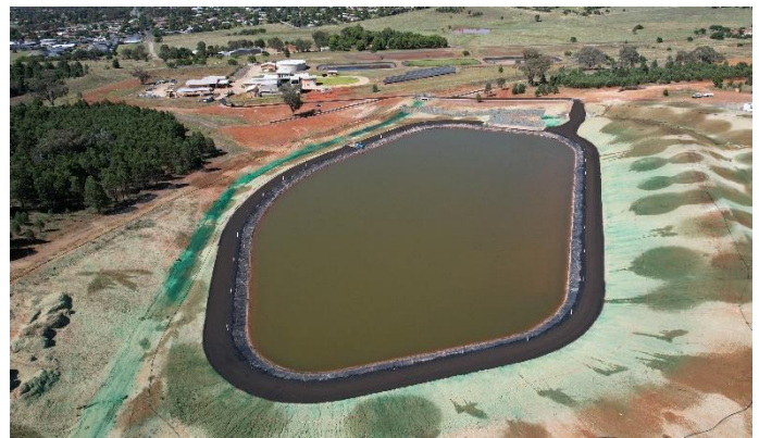
Figure 1: The RWSL has been completed, following the application of hydro-mulching around the batters of the lagoon.
