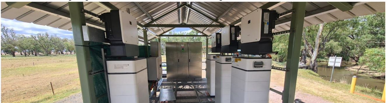
Figure 2: The batteries and inverters for the solar array have been installed at the Lachlan River Precinct.
